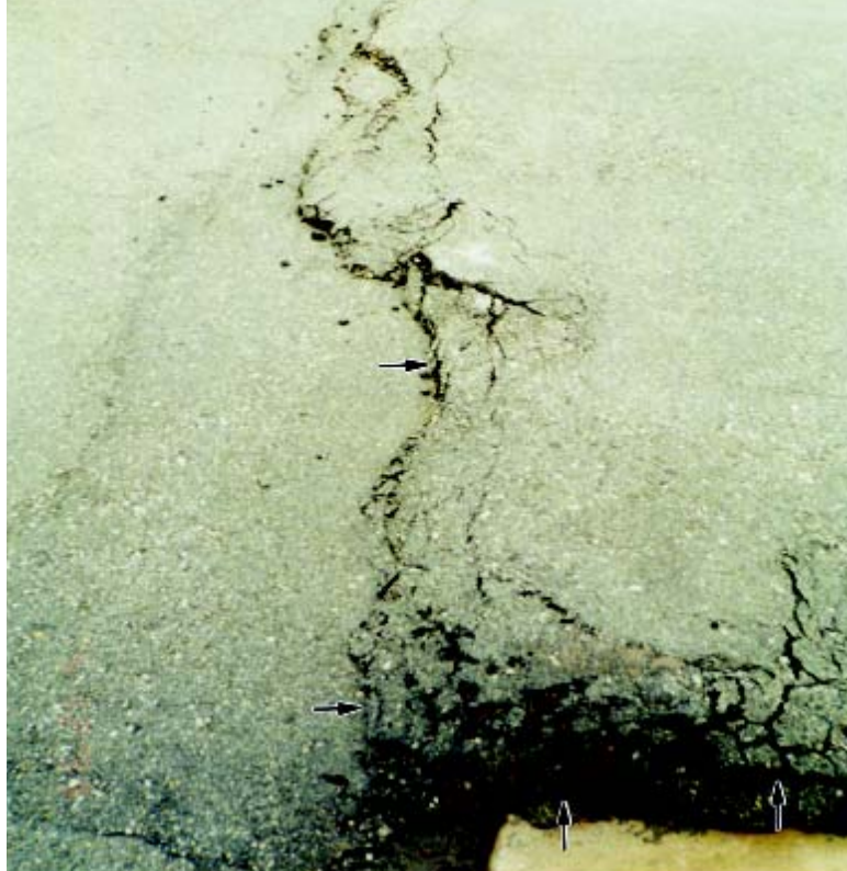
Fig. 2: Asphalt distortion at Runway 12R-30L
