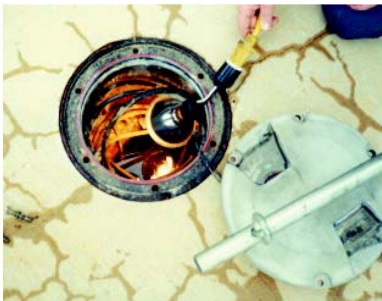
Fig. 3: An affected light base in the runway in which the Touchdown Zone Light circuit cable had severed
