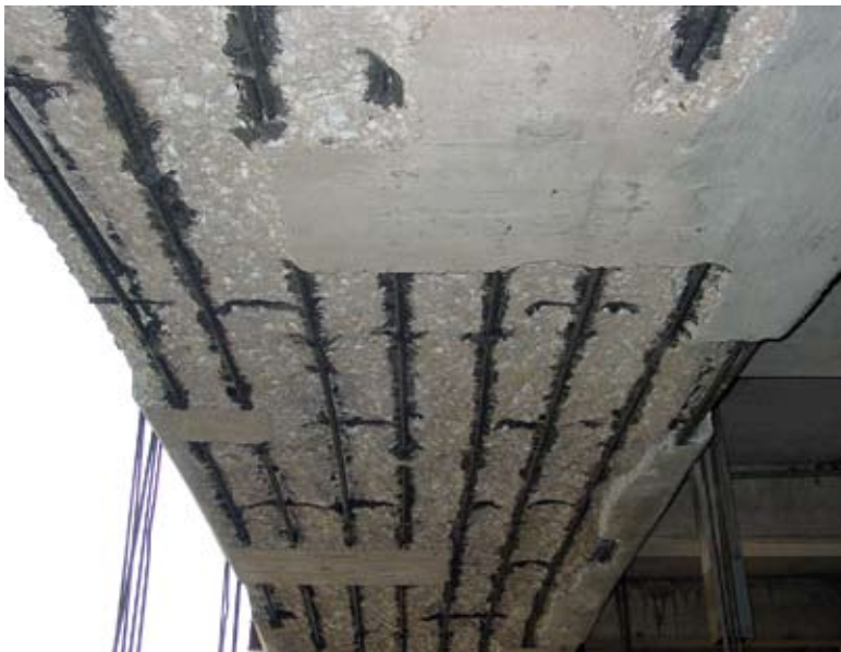
Severe corrosion of bridge arches
