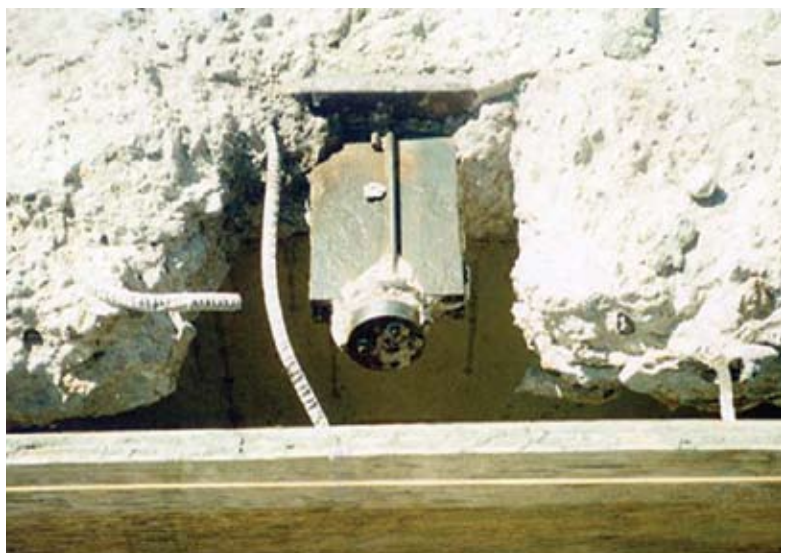
Fig. 4: View of exposed button-headed tendon anchor. Note failed wire on top side of spacer/shim plates
