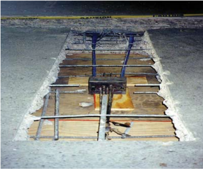
Fig. 6: Typical splice arrangement between single button-headed tendon and two monostrand tendons. Photo depicts arrangement at non-stressing end
