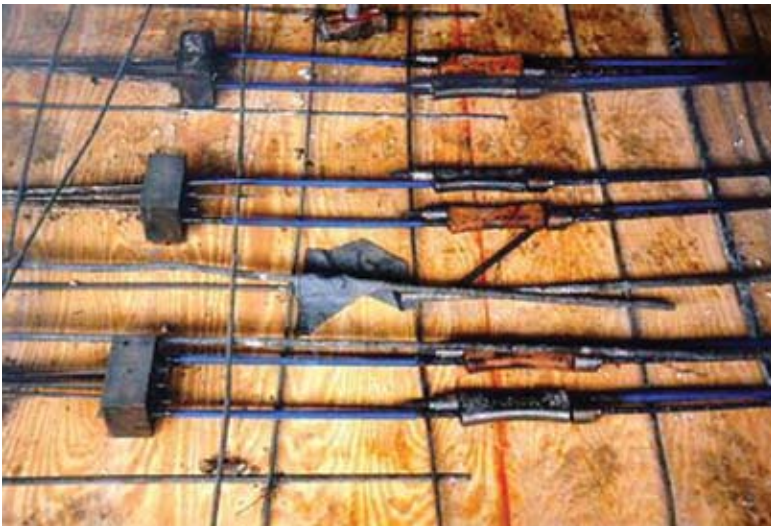
Fig. 7: Tendon splice arrangement with multiple adjacent tendons. Note splice transition block between single B/H tendon and two monostrand tendons, as well as dogbone stressing anchors
