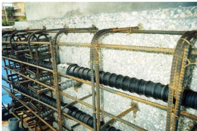
Fig. 10: Bursting steel around spin-lock anchors, two horizontal post-tensioned tendons, reinforcing steel dowels, and reinforcing steel cage
