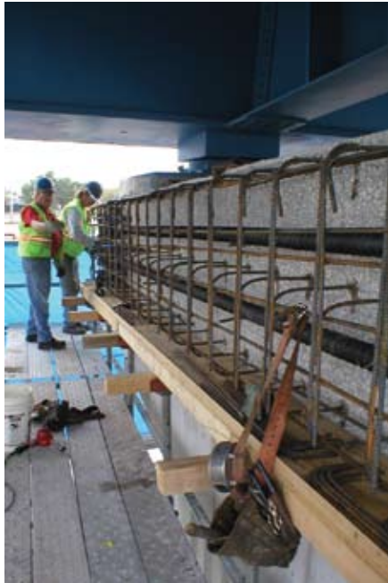
Fig. 4: Installing reinforcing steel cage and bursting steel around post-tensioned tendons on Pier Three
