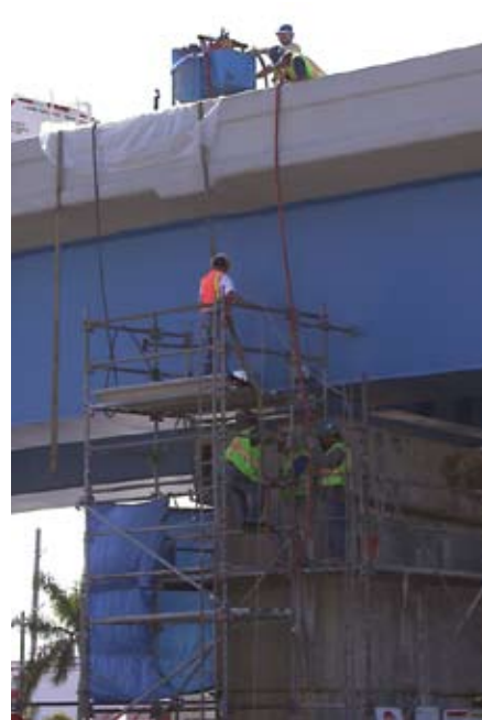
Fig. 6: Grouting post-tensioned tendons from colloidal mixing operation staged on top of bridge
