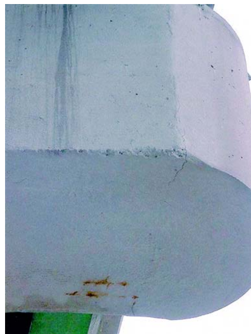
Figure 2: Detail of the pier cap from the west, showing cracks
