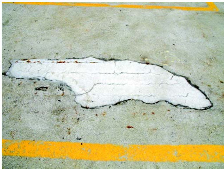
Fig. 1: Patch repairs like this one are all too common
