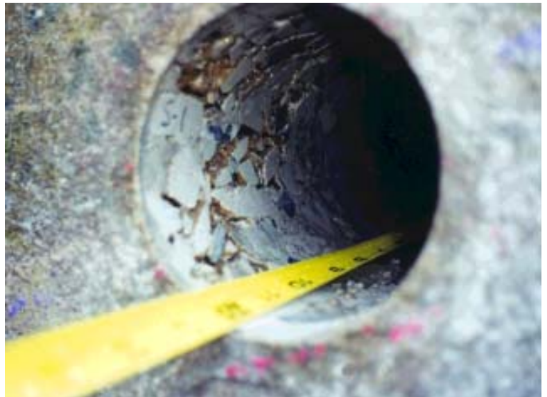
Fig. 7: Poor consolidation detected by IR testing, even though concrete surface was sound
