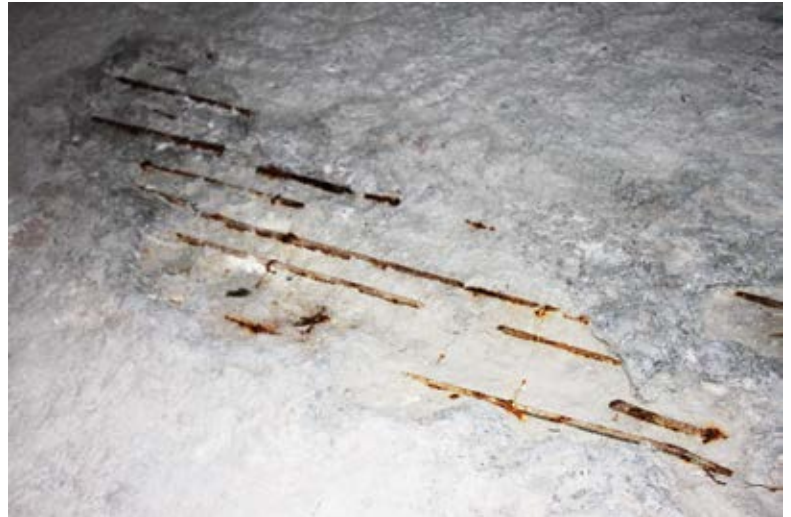
Fig. 4: Water infiltration reached the reinforcing steel, causing corrosion
