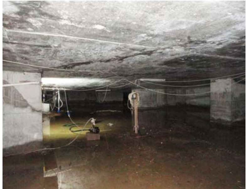
Fig. 3: The originally specified surface-applied membranes failed at below-grade levels, causing severe leakage
