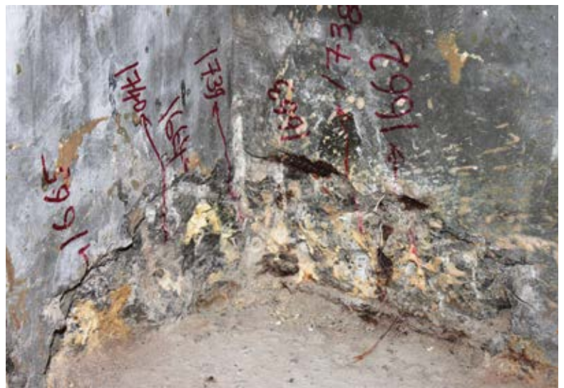
Fig. 5: The injection method was attempted many times without success, increasing costs, and delaying the project schedule
