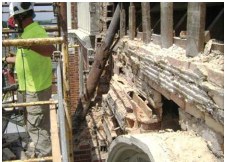
Fig. 7: 1920 construction consisted of a variety of load-bearing materials including cast stone, hard- and low-fired brick, terra-cotta tile, steel, hard dense pointing mortar, and lime sand mortar
