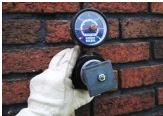
Fig. 8: Anchorage testing—two tests should be performed: one on the backup material and another on the brick or mortar at the exterior veneer surface. Without these two independent tests, verification of the veneer holding system is inadequate
