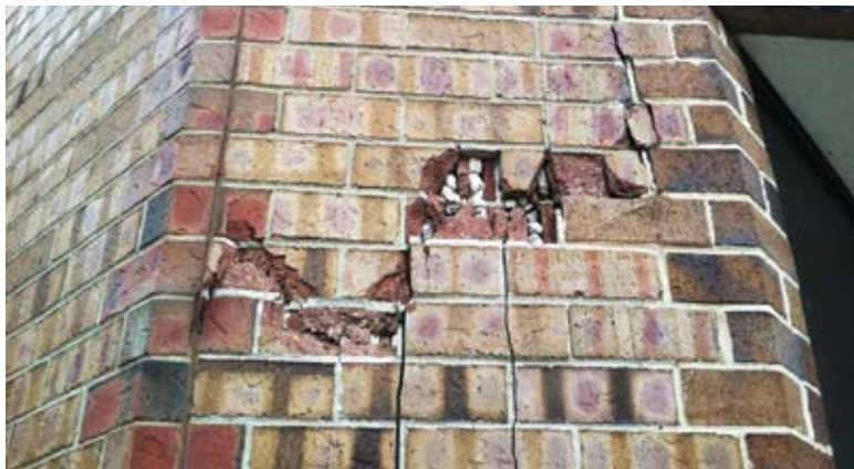
Fig. 2: Above this vertical shear in the brick masonry, 200 ft (61 m) of jumbo brick wall moved both vertically and horizontally, requiring immediate shoring and investigation for permanent repairs
