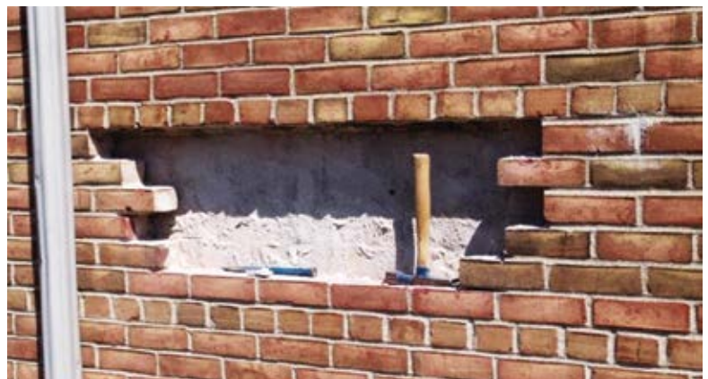
Fig. 6: Destructive removals of the veneer system found that the backup structural block system was parge-coated during construction for waterproof integrity. The tie brick was actually inserted into the block wall system
