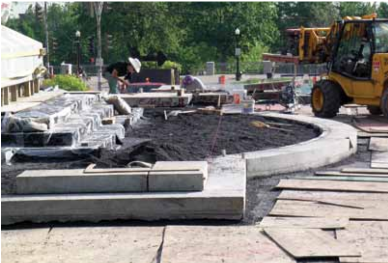
Reinstallation of granite blocks on crushed scoria Photo courtesy of the city of Montréal
