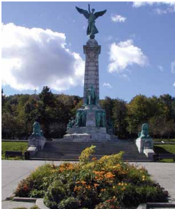
Sir George-Étienne Cartier monument before restoration Photo courtesy of the city of Montréal
