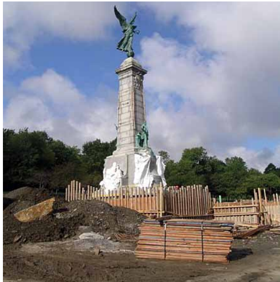
Cofferdam at the base and protection of the obelisk with wood and straps, spring 2006 Photo courtesy of the city of Montréal
