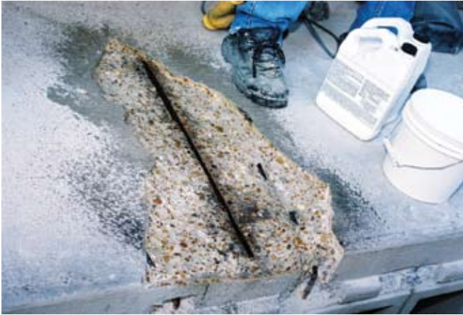
Patch prior to repair
