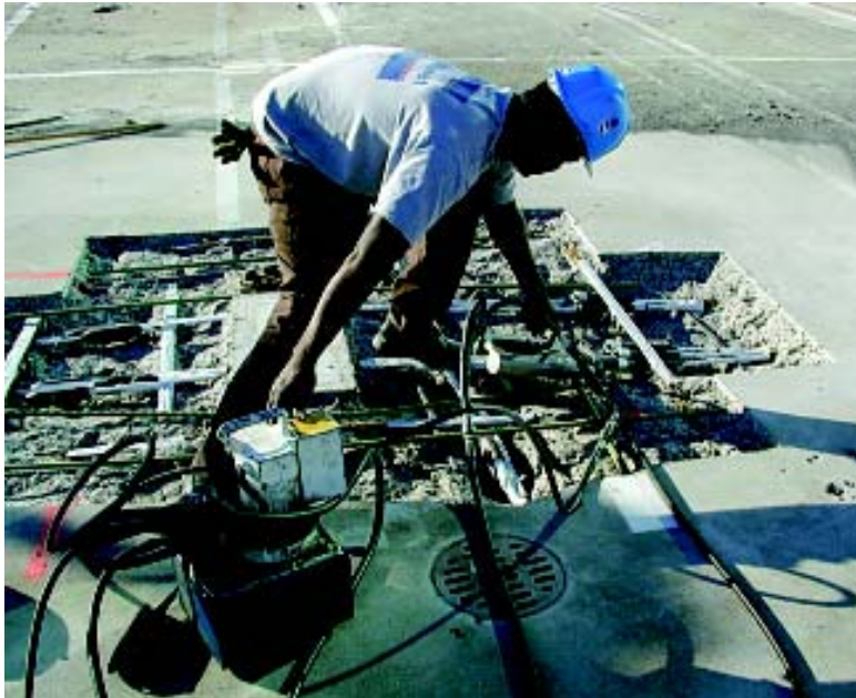
Fig. 1: Repair to a two-way flat plate parking structure built in 1971. Two-way structures built during the 1960s and 1970s often used a “basket-weave” tendon layout; tendons were distributed in both directions. Current practice is to band the tendons in one direction
