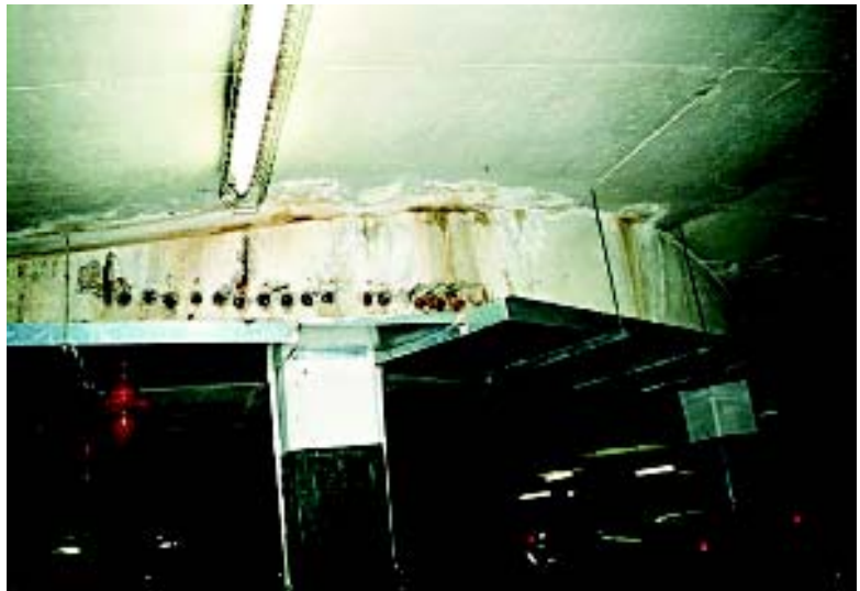
Fig. 3: Water leaking from an open construction joint at a slab/wall joint has severely corroded all of the anchors in this band. Several of the anchorages have failed. Drip pans have been installed along the length of the joint
