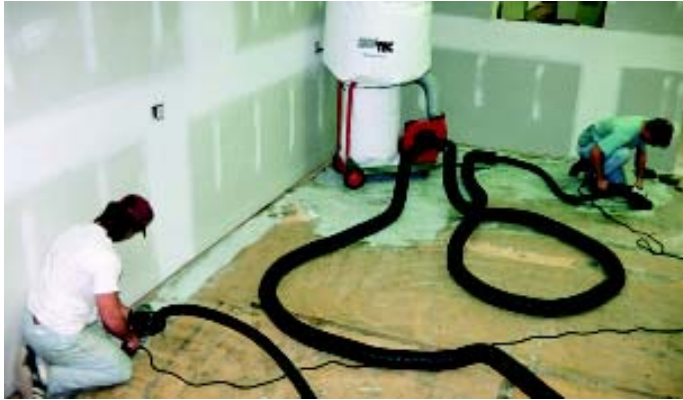
Some hand work is frequently required; use of dustless equipment protects workers and keeps the surrounding areas clean.
