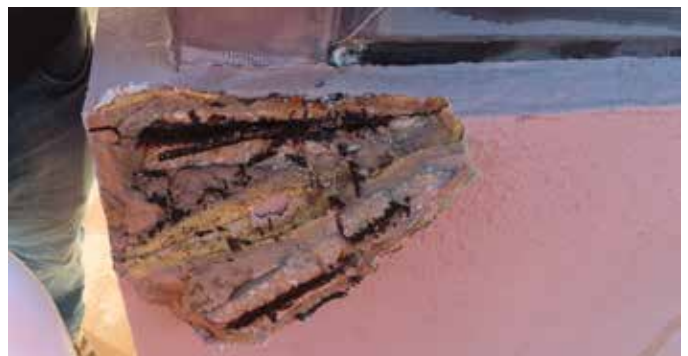
Fig. 4: Concrete spall due to corroded reinforcing steel at precast concrete window sill
