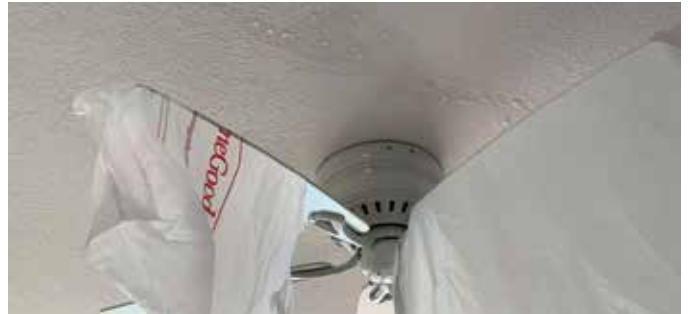
Fig. 2: Water intrusion from Hurricane Eta adjacent to the ceiling fan
