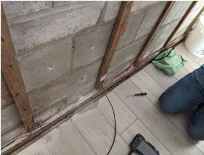
Fig. 5: Investigative exploratory opening inside condo unit revealing water intrusion
