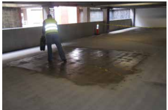
Fig. 8: Application of surface-applied corrosion inhibitor to parking garage surface at test area showing sectioned installation for ensuring adequate coverage rates
