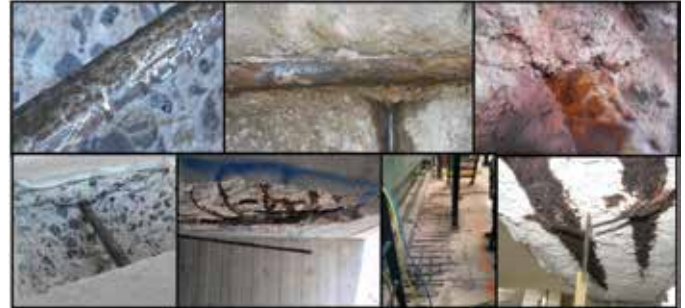
Fig. 3: Corrosion-related distress: (a) pitting from chloride-induced corrosion (after bar cleaning), (b) corrosion products compared to bare steel, (c) corrosion-induced cracking, (d) cross-section of delamination, (e) overhead delamination and spalling hazard, (f) horizontal spalling and tripping hazard, and (g) reinforcing steel disintegration
