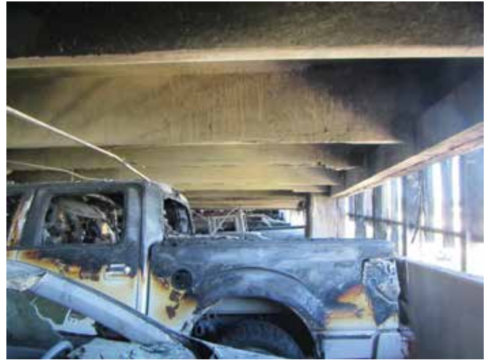
Fig. 2: Fire damage on Level 3 of parking garage
