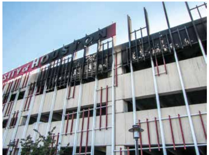
Fig. 3: Fire damage at exterior of garage
