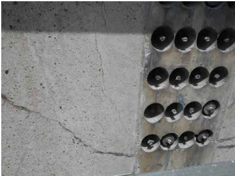
Fig. 8: Shear cracking at post-tensioned cable anchorage
