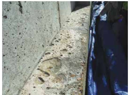
Fig. 3: Honeycombing damage on concrete beams
