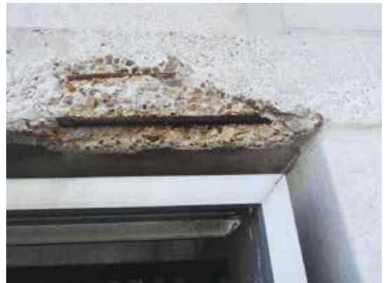
Fig. 2: Major spall due to rebar corrosion on building façade
