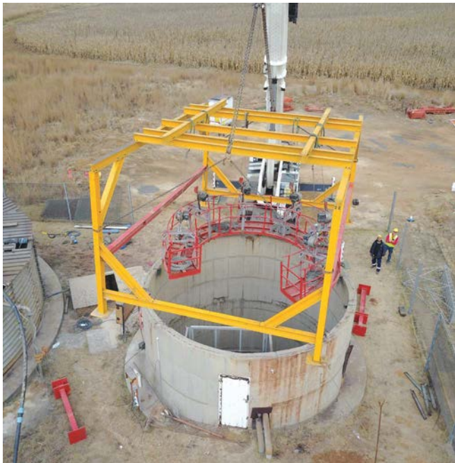
Fig. 3: Access to the shaft was a huge safety and logistical concern. The access specialists were able to supply a custom-built cradle to lower workers into the shaft. This cradle was anchored to the sides of the shaft to ensure no movement during the high-pressure cleaning and sandblasting.
