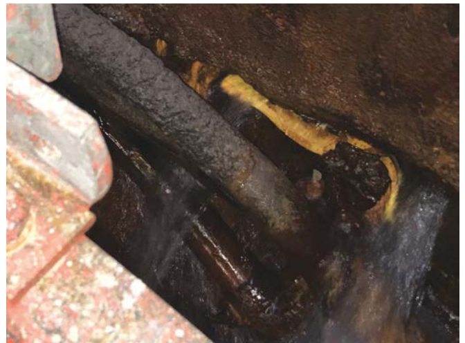
Fig. 5: The waterproofing specialists tested the swelling waterstop on the ingress points to ensure the waterstop would swell to its maximum capacity to alleviate water pressure to continue with the crystalline leak repair system.
