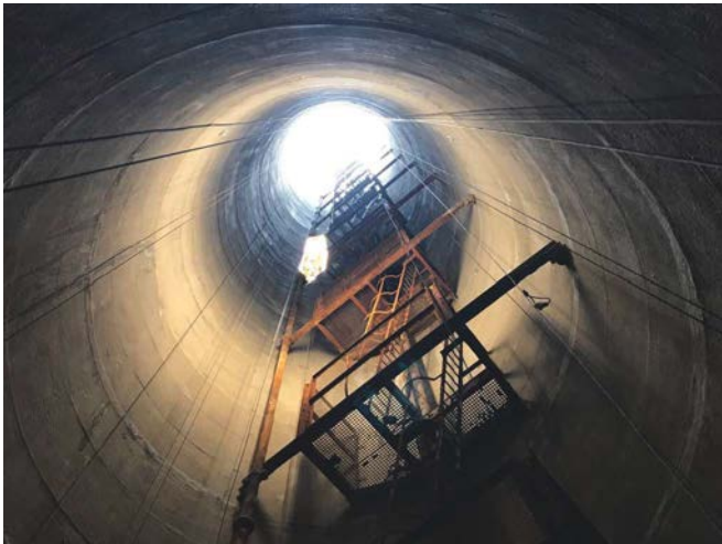
Fig. 8: View from the bottom of the shaft once the project was complete
