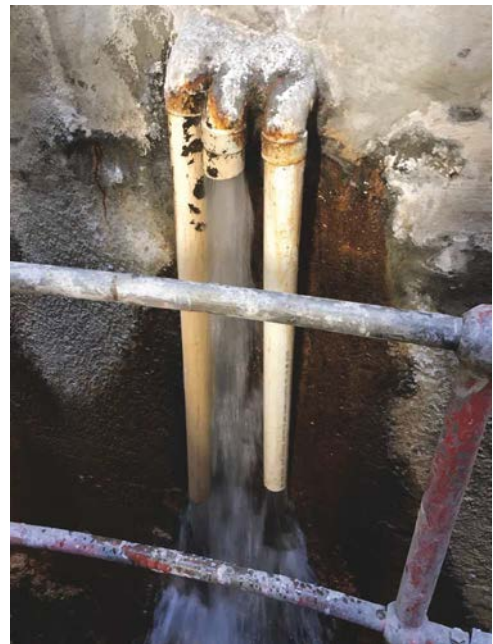
Fig. 6: Using a rapid-setting hydraulic cement and a swelling waterstop, the waterproofing specialists were able to successfully contain the flow of water to a single access point, thus making the water more manageable.
