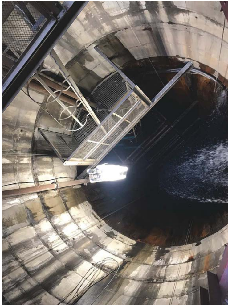
Fig. 1: View from the top of the shaft during the site inspection. The extreme water ingress points are evident all the way down the ventilation shaft. The base of the ventilation shaft was filled with water for 35 years.
