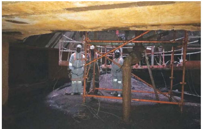
Fig. 9: The base of the shaft had not been seen or dry for over 35 years. This was the first time that workers were able to stand at the base of the shaft.
