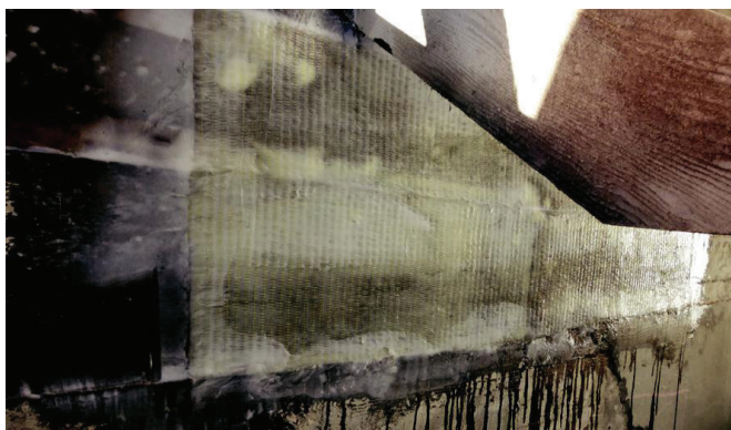
Fig. 9: Repair application of FRP at horizontal joint prior to new parge coat
