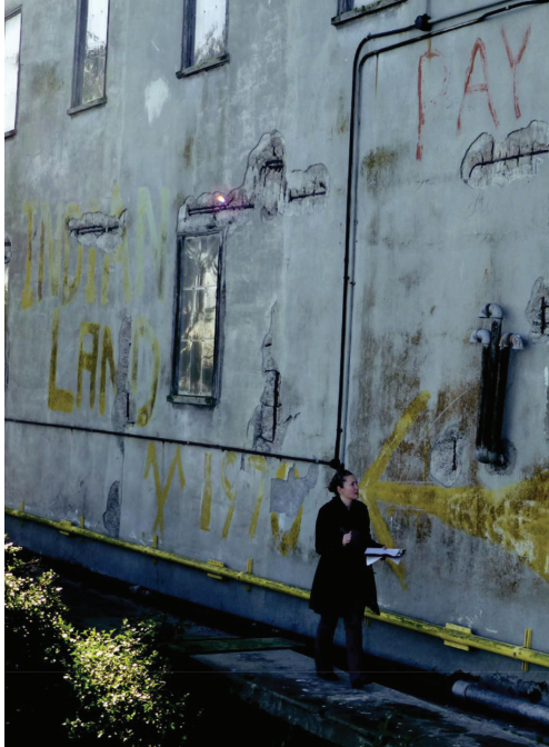
Fig. 11: Close-up view of deterioration at location of political statement in Figure 10
