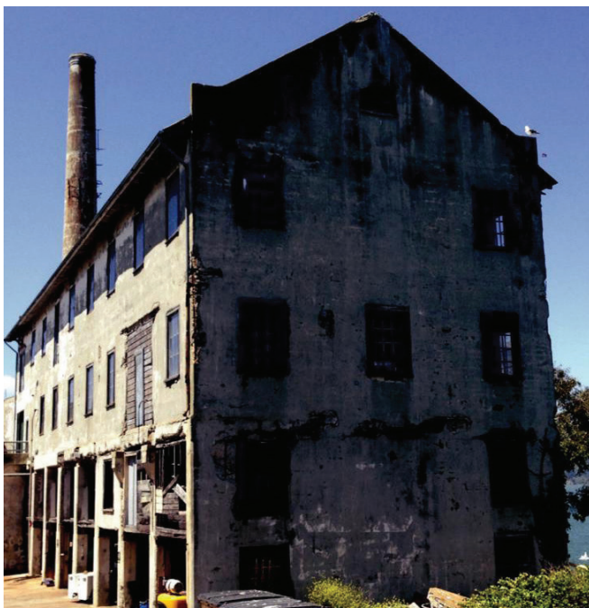
Fig. 4: Deteriorated Quartermaster Building, circa 2013 (prior to restoration)
