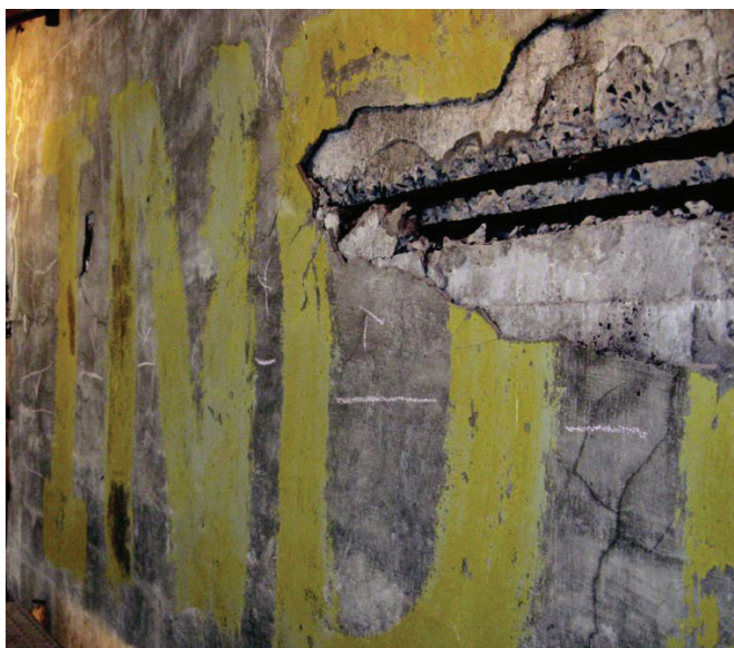
Fig. 10: Deteriorated conditions at locations of political statement in 2014 (prior to repairs)
