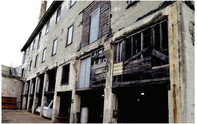
Fig. 5: Deteriorated Quartermaster building in 2016 (prior to restoration)
