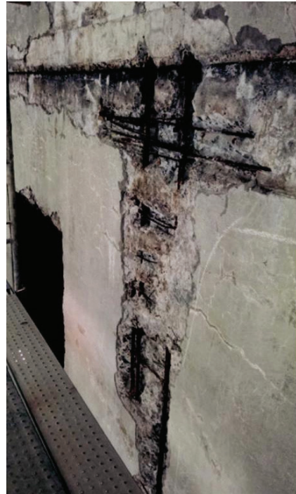
Fig. 6: Exterior concrete deterioration in 2016 (prior to restoration)
