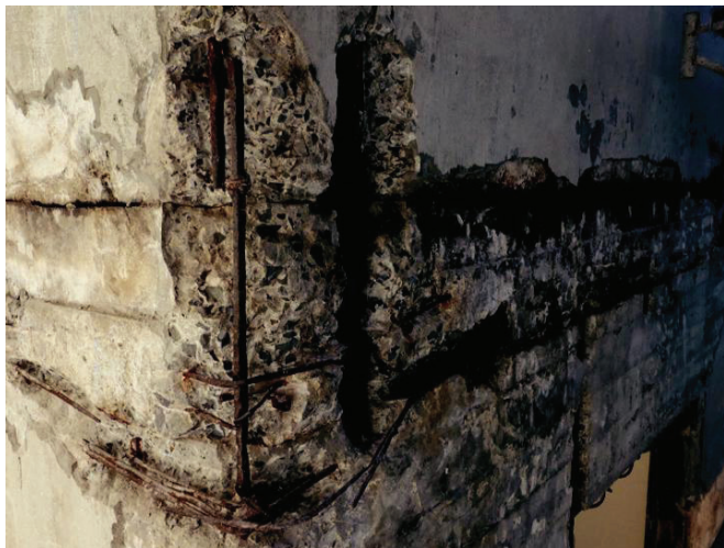
Fig. 8: Cold joint revealed during parge coat demolition
