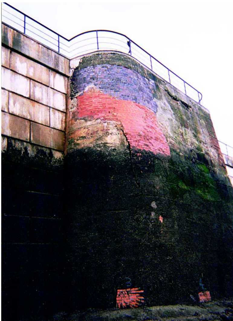
Figure 3: Previously repaired area
