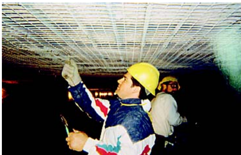
Fig. 7: Placing 2 in. x 2 in. galvanized welded wire fabric over reinforcing to aid in build-up of shotcrete material and to make the repair monolithic with the substrate
