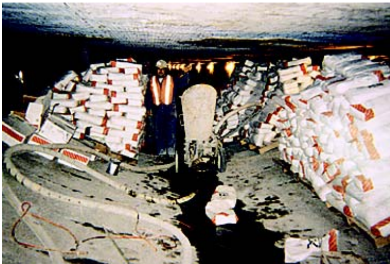
Fig. 4: Work done under roadway. All shotcrete material came in 50 lb bags which were transported to the project location by hand through manholes
