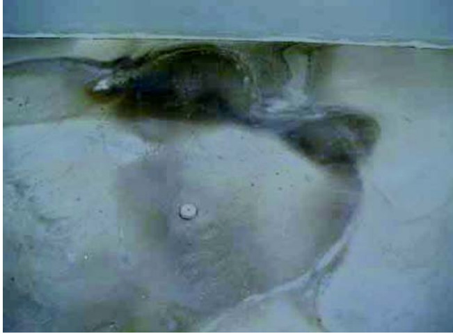
Mottling appearance of the underlayment characterized by overwatering, improper mixing, or both
