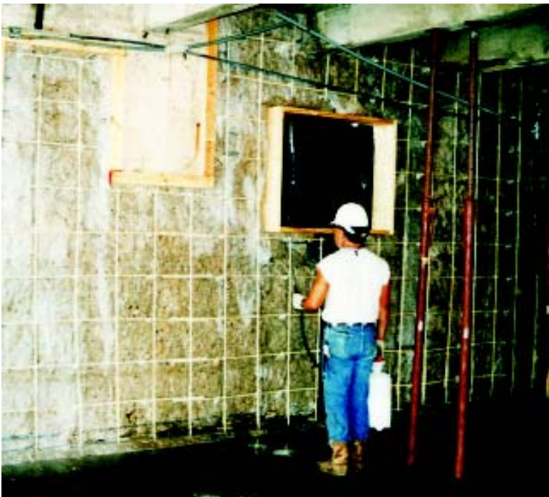
Figure 4: Application of bonding agent to concrete behind new fiberglass reinforcing prior to shotcreting
