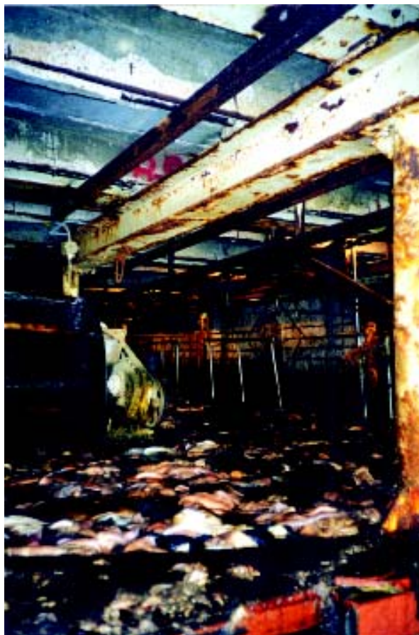
Figure 2: Beam deterioration over hide vat
