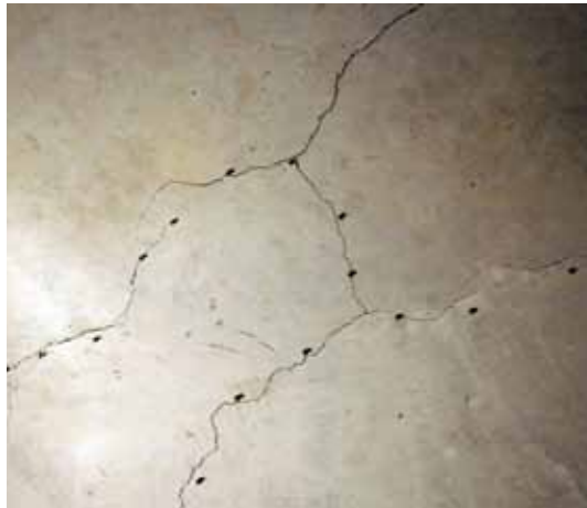
Existing condition—cracks on underside of garden level slab
