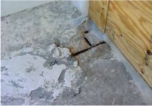
Corrosion of reinforcement along the internal edge of the balcony created great concern for future damage to the interior of the condo unit
