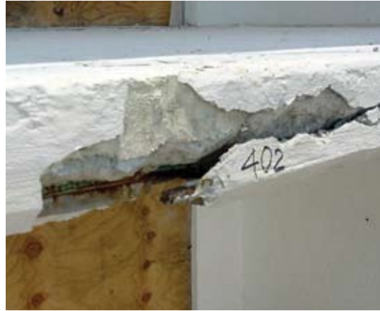
Typical spall on underside of balcony edge
