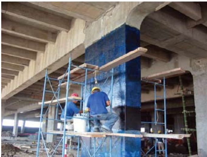
Fig. 5: Carbon-fiber bands were used to wrap adjacent columns and to ensure that the 15 blocks behaved like one unit
