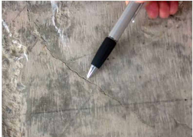
Fig. 3: Diagonal cracking on the columns
