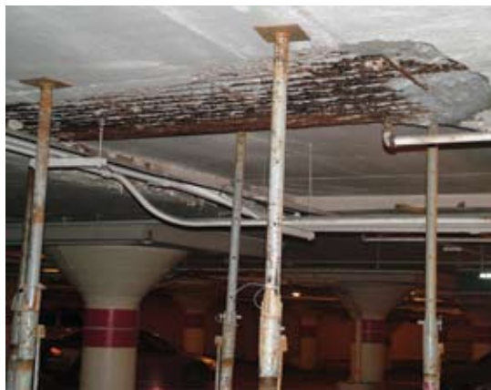
Delaminated soffit repairs
