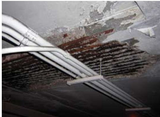
Existing soffit corrosion (note the electrical conflicts/challenges)
